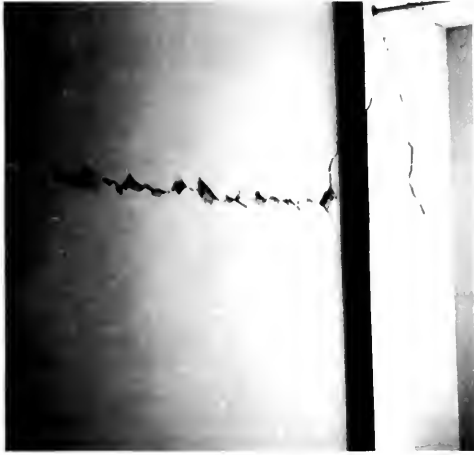
Photo 4. Los Angeles High School. Interior-partition damage at stairway.
